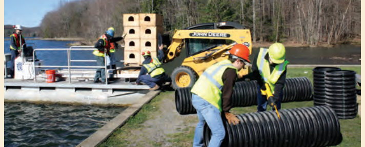
In front, left to right, Penn State DuBois Wildlife Technology Students Alec Baker and Teanna Kobuck cut section of corrugated pipe to be used in the construction of catfish spawning boxes, as other sections of the artificial habitat are loaded onto a pontoon boat behind them.
